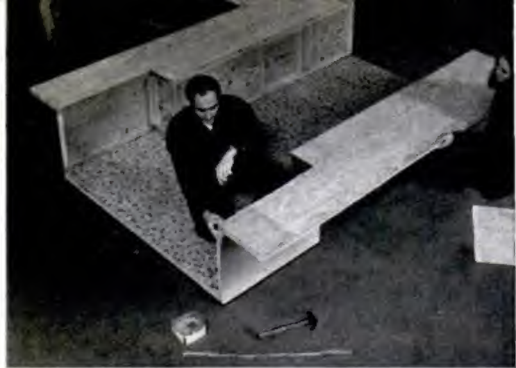
CAMPER-FLOOR BASE is completed and covered with linoleum. Next, wall sections are fastened to the base
